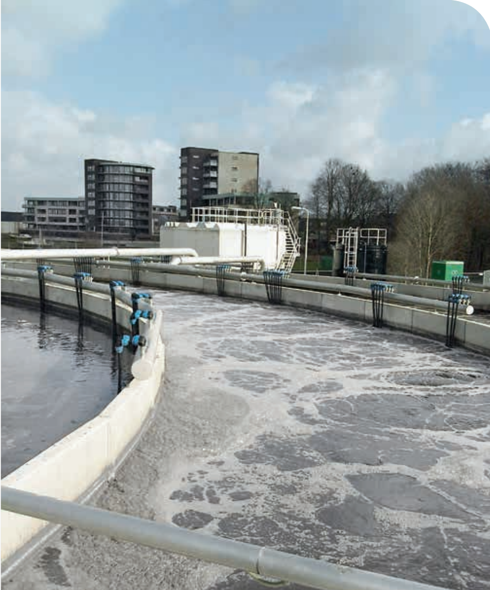
Wastewater treatment plant Steenwijk, Netherlands
